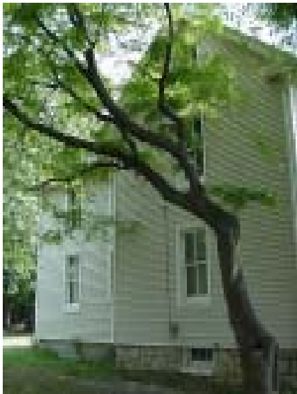
Re-siding the entire house helps the facade of the rear addition blend in smoothly with the original structure.
